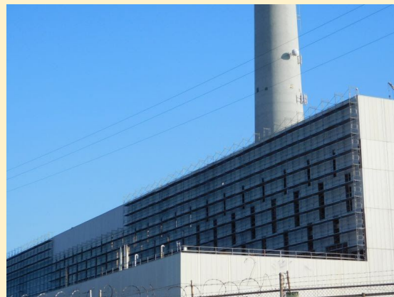
Scaffolds on the front face of the Power Plant are used to remove concrete panels (CHS- GG)
