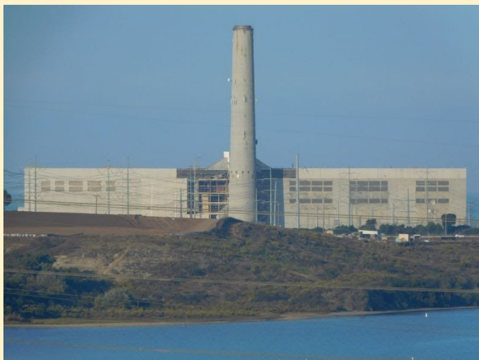
Panels have been removed from the back of the Power Plant (CHS-GG)
